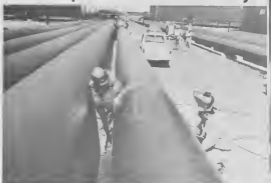
Welders P. Simileer (left) and L. de Cuba working on the 36-inch pipeline which is over 5000 ft. long.
